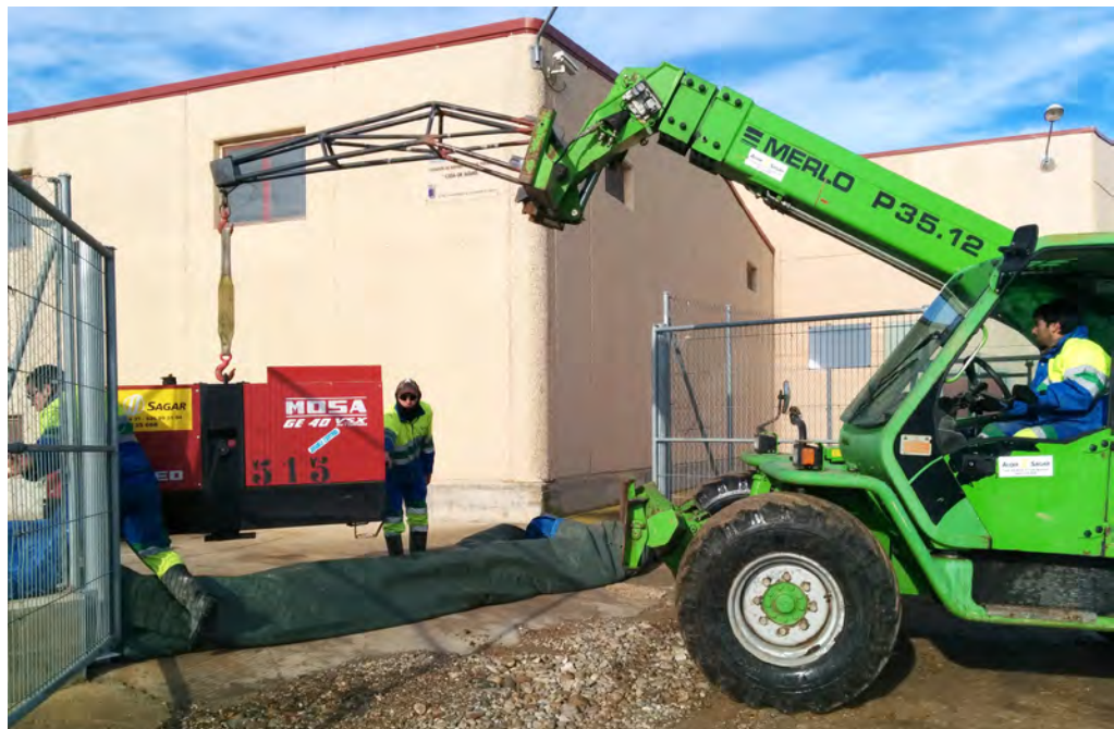
In the photo, a scene when, following the contingency plans, the ancillary equipment is introduced in the Calahorra Drinking Water Treatment Plant.
